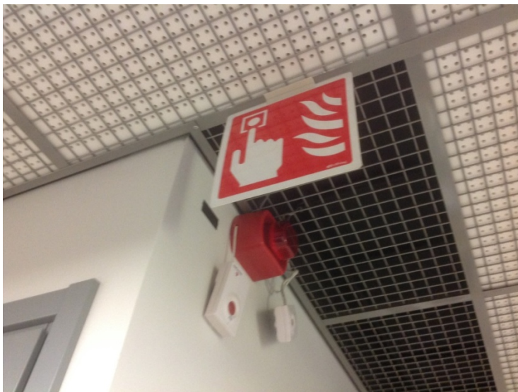
Fig. 4. A clear visual signal in the ceiling, if there is a general alert. There is also a loud siren type sound involved for the hearing impaired. This is also connected to employers' vibrating alert pagers.
