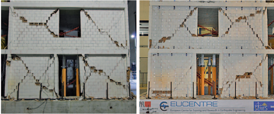
Fig. 18.11 Damage in the URM piers of the first two storeys after test number 9
