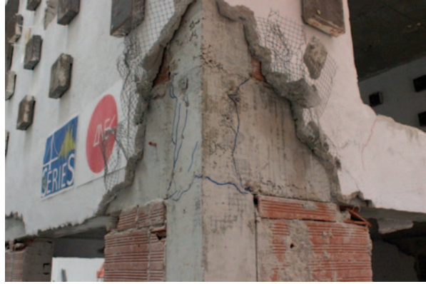
Fig. 16.12 Extensive cracking observed upon reinforced coating removal at the beam-column connection in the Northwest corner
