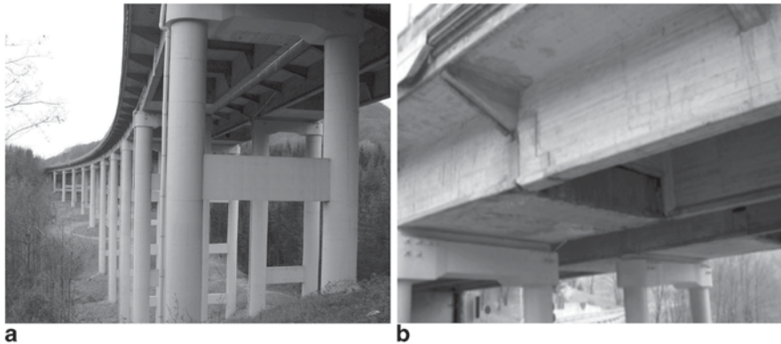
Fig. 7.1 a Views of the Rio Torto viaduct portal piers. b Views of the Rio Torto viaduct concrete decks
