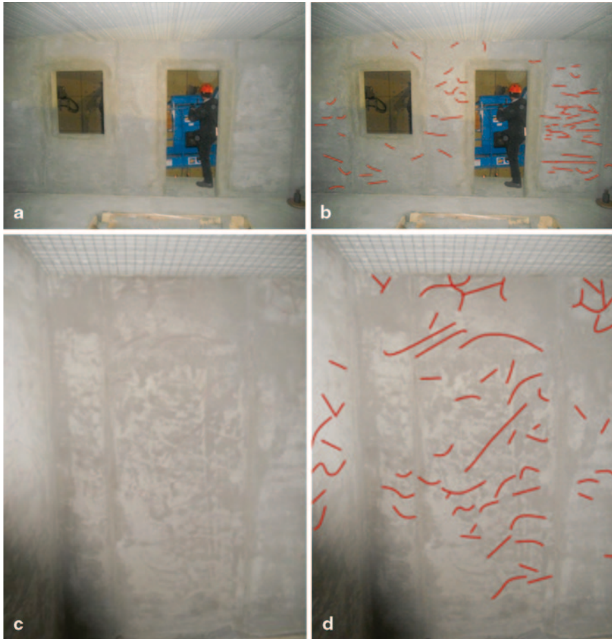
Fig. 21.7 a and c Cracking pattern after the 0.5 g white noise (inside third floor) b and d same walls with cracks underlined in red
