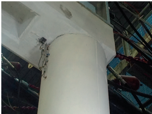
Fig. 14.17 Crack opening at the top of a column in the short pier after test k12 (PGA=200% ULS)
