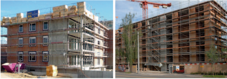
Fig. 18.1 3- and 8-storey residential buildings with RC walls and URM walls. (Reproduced by permission of Thomas Wenk)
