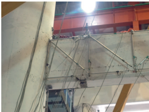
Fig. 14.19 Crack pattern in the first transverse beam of tall pier after test k12 (PGA=200% ULS)
