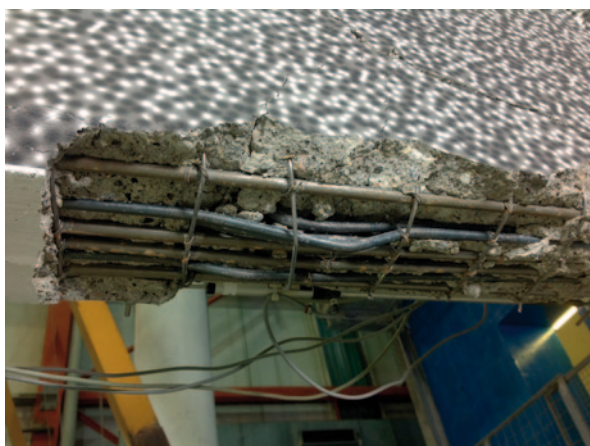
Fig. 14.18 Blow up of the transverse beam damage on short pier after test k12 (PGA=200% ULS)
