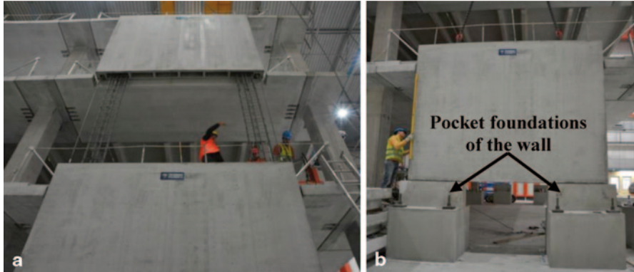
Fig. 24.2 a Assembling phase of the precast walls. b Pocket foundations used for the walls
