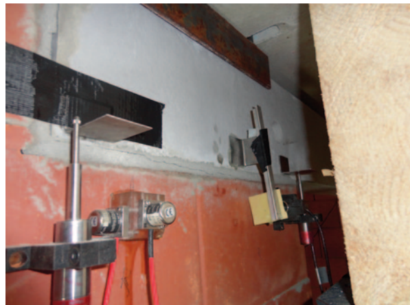
Fig. 17.14 Cracking of the lintel supports
