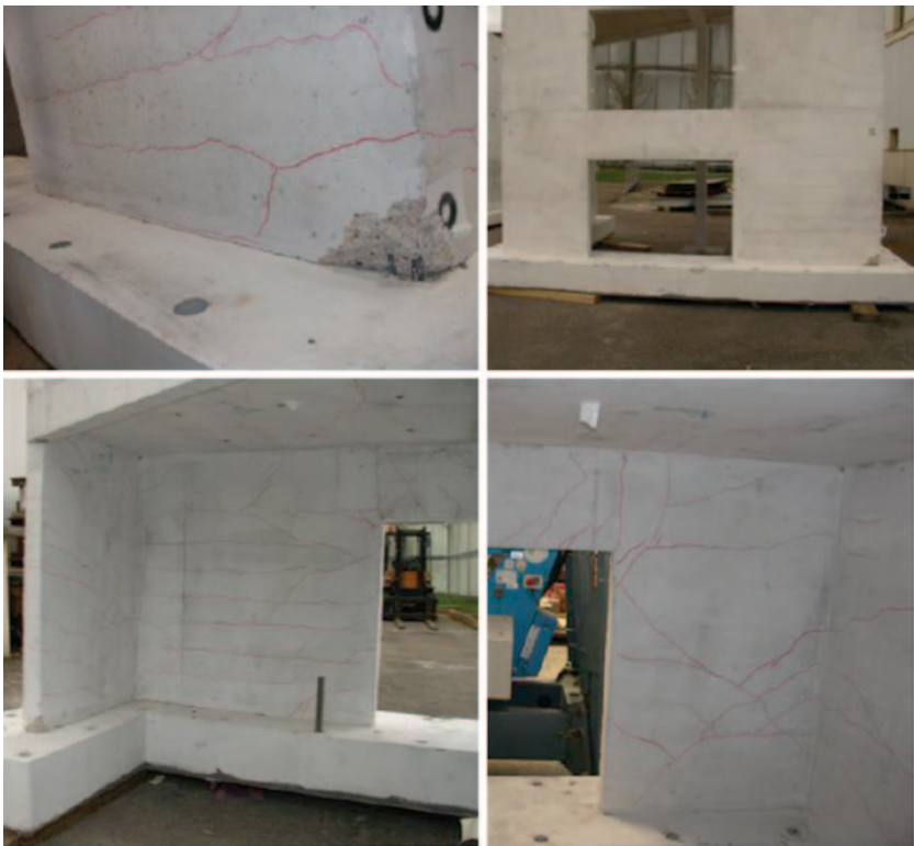
Fig. 19.17 Damage observed on wall 2 after the tests
