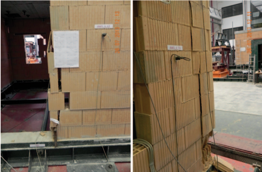
Fig. 15.10 Local failure of asymmetric Mock-up B
