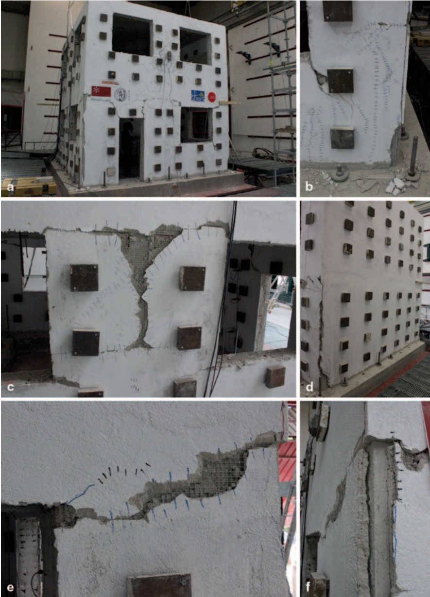
Fig. 16.11 Damage after additional seismic tests a North façade, b crack and mortar coating loss at the Northwest corner, c crack at the interior jambs in the infill wall at the ground floor of the East façade, d South façade, e crack at the a lateral jamb in the infill wall at the ground floor of the East façade, f crack and mortar coating loss at Northeast corner
