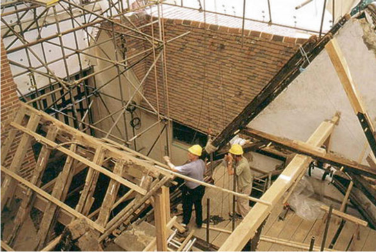
Fig. 7.1 The major repair project at Ightham Mote, Kent (UK), undertaken on behalf of the National Trust, had the benefit throughout of an archaeologist working alongside the architect and contractor to inform the process and record what was discovered (Photo: Jason Wood)
