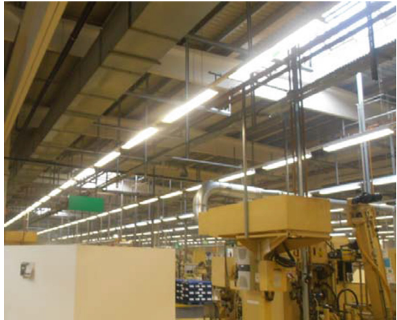
Fig. 2 Picture that shows the layout of the lighting installation in the production hall analyzed
