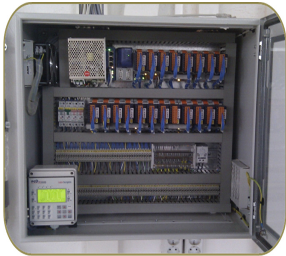
Fig. 5 Electrical board of the data acquisition and processing system
