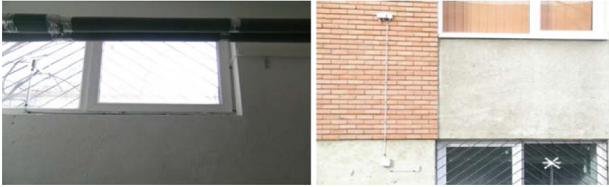
Fig. 6 Temperature sensors that have been mounted on the inner and outer surfaces of the wall and window
