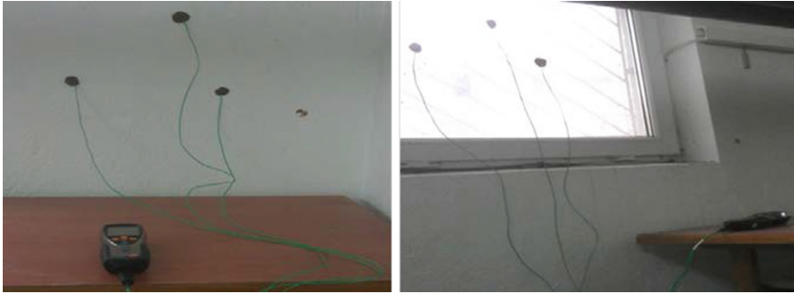
Fig. 4 TESTO sensors mounted on the inner surface of the exterior wall and window
