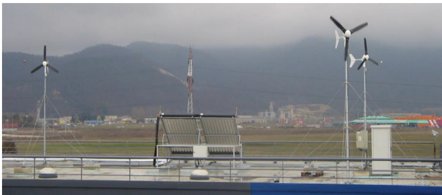
Fig. 6 Three wind turbines of 300 W each, installed on the terrace of one of the Research Institute buildings
