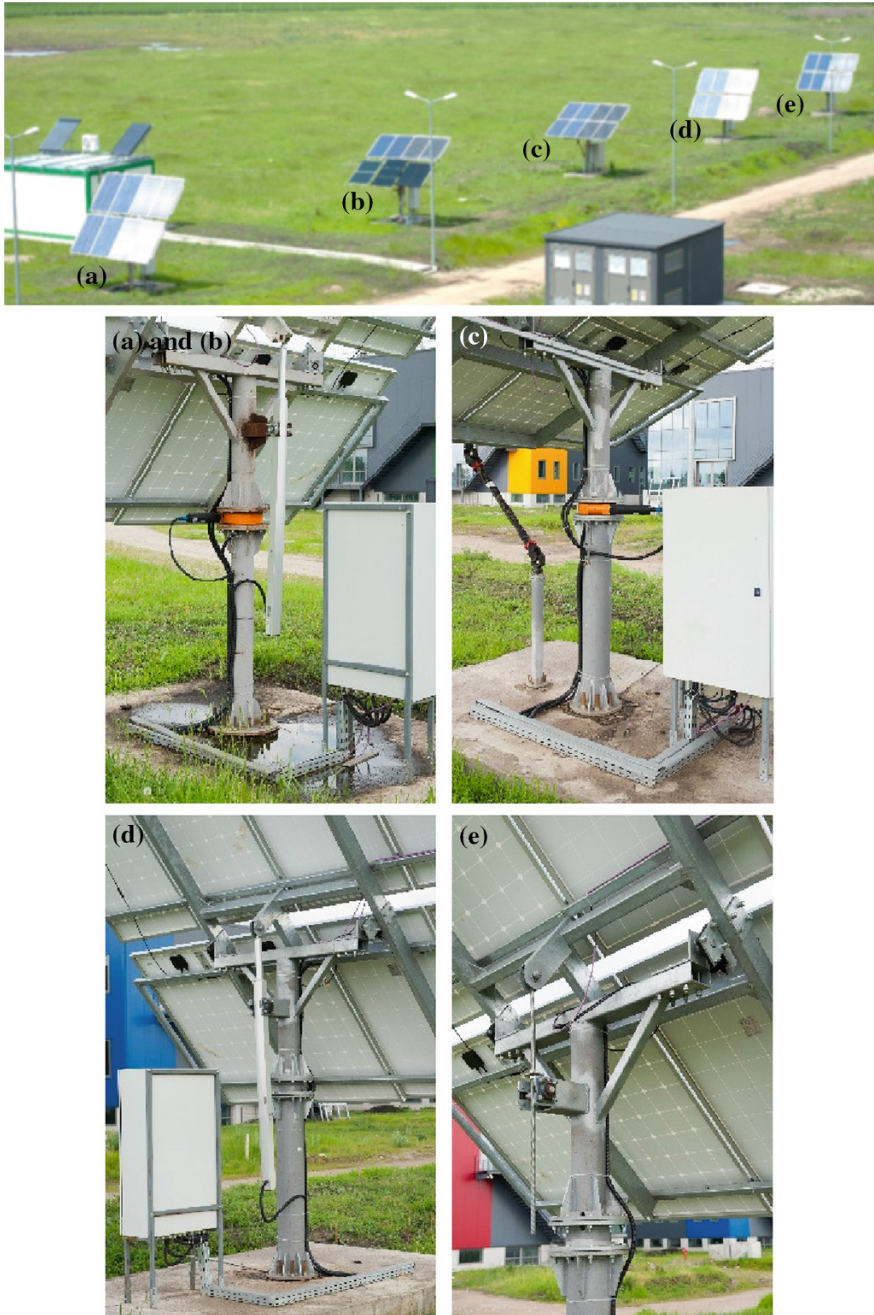
Fig. 10 Tracked PV platforms for implementation close to the buildings: general view and tracking systems: a and b azimuthal biaxial tracking systems with actuators; c azimuthal, biaxial tracking system with universal joint; d monoaxial tracking system with driven elevation control, and e monoaxial tracking system with manual system for elevation control
