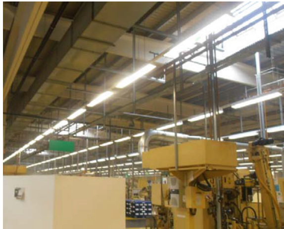
Fig. 2 Picture that shows the layout of the lighting installation in the production hall analyzed
