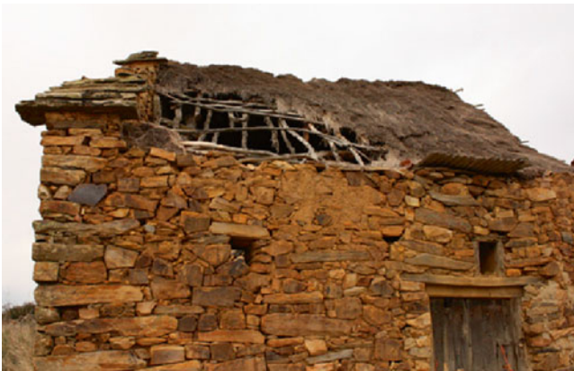
Fig. 3.3 An abandoned vernacular house made of stone, wood, and straw, inhabited until the 1980s
