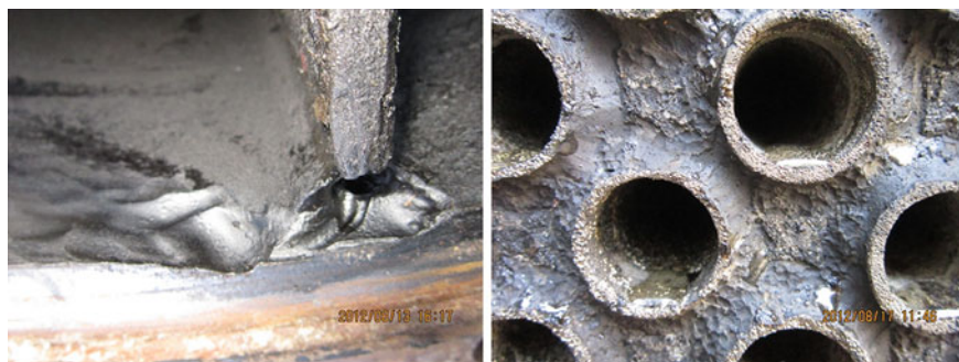
Fig. 2 Erosion-corrosion at the junction of channel flange and partition plate of E119A ( left figure ), corrosion of tubes and tubesheet of E112A ( right figure )
