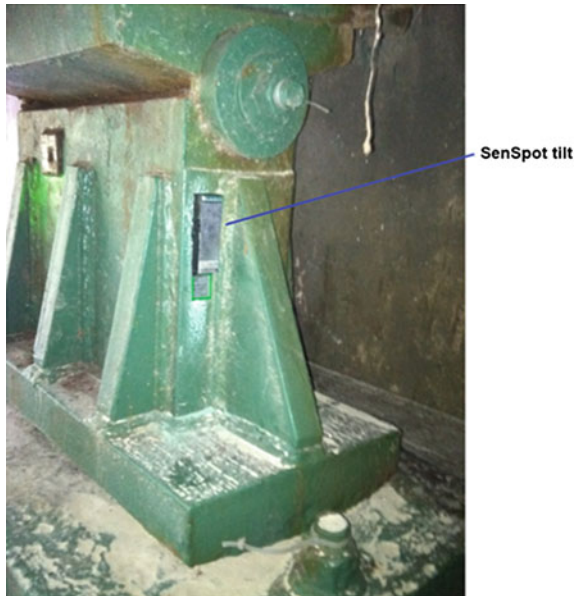
Fig. 4 Wireless tilt sensor on a rocker bearing of a highway bridge
