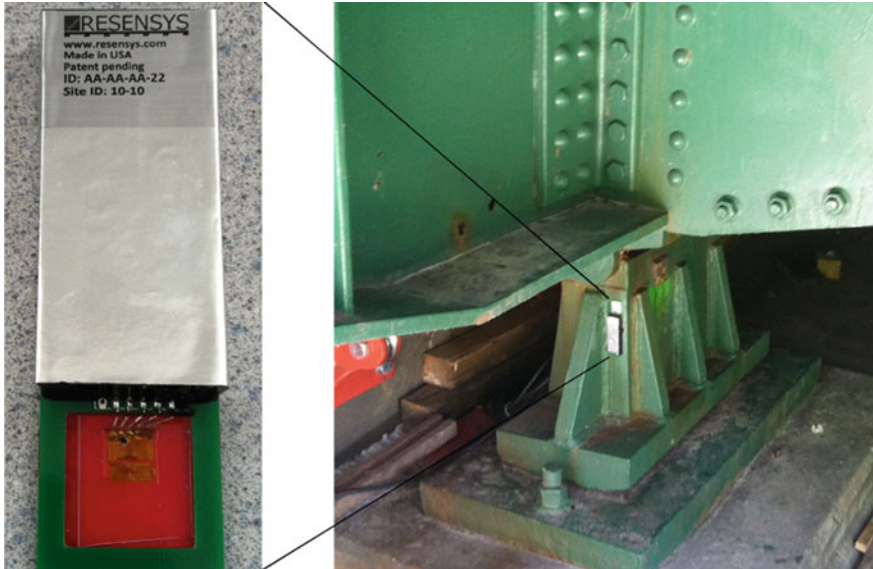
Fig. 1 Resensys SenSpot ( left ) and installed sensor on a bridge bearing ( right ) for tilt and loading monitoring
