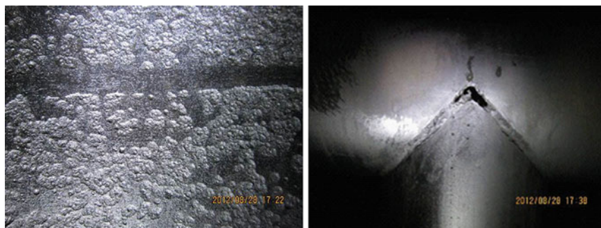
Fig. 1 Pitting corrosion of tower wall, fillet welds penetrated corrosion distributor pipeline at vacuum side cut 3 back to tower
