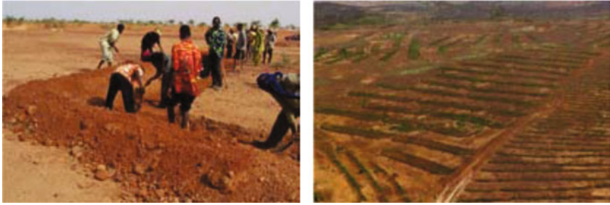
Fig. 16.3 Construction of contour bunds ( left ). Rows of contour bunds ( right ) (Source: GIZ 2012)
