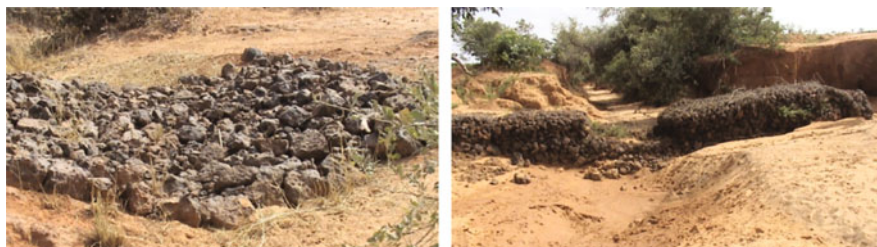
Fig. 16.5 Closing-off of a gully with permeable rock dam ( left ). Treating a gully with gabion ( right )
