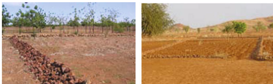
Fig. 16.2 Construction of rock dikes ( left ). A series of rock dikes in a field ( right ) ( Source: GIZ 2012 )
