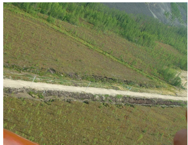
Fig. 58.3 Dangerous site with thermoerosion on the polygons with ice wedges along oil pipeline "Eastern Siberia–Pacific Ocean-1" (ESPO-1) in Chulman area
