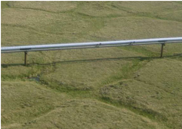
Fig. 58.1 Ice wedge polygon in shape of a regular square on the Badami oil pipeline in northern Alaska (Fiscal Year 2007 lease compliance monitoring report)
