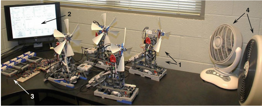
Fig. 14.1 Wind farm general view: (1) wind turbines; (2) SCADA and central control system; (3) smart micro grid with batteries, electrical loads, switches and solar panels; (4) fan system
