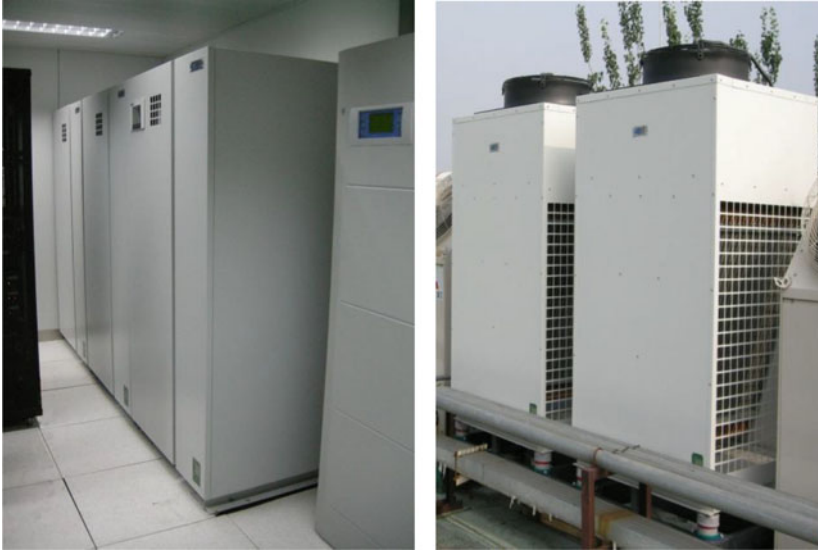
Fig. 40.9 HPCS of the data center in Beijing
