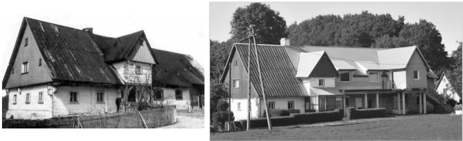
Fig. 9. An unsupervised extension of a 19th century cottage eliminated the original features of the house: on the left – the original form as of 1996, on the right – the same building as of 2012 with a new reinforced-concrete porch (Wilkanów) (photos by E. Trocka-Leszczynska)
