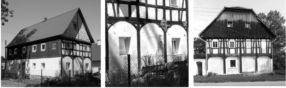
Fig. 7. Amateur renovations: on the left and in the center – the wooden walls of the ground floor and gable have been walled up (Wlosien 2006), on the right– the wooden structure of the round floor has been walled up (Bratkow) (photos by E. Trocka-Leszczynska)
