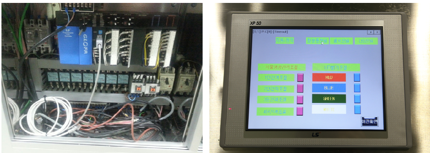
Fig. 6. Installed PLC and Controller in Proposed Intelligent Plant Factory System
