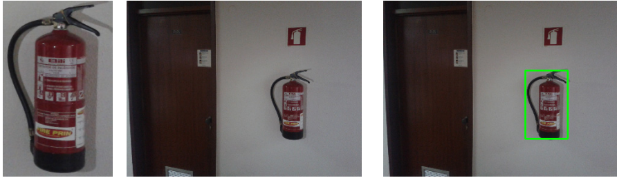
Fig. 5. Detection of fire extinguisher in the corridor (case #2)
