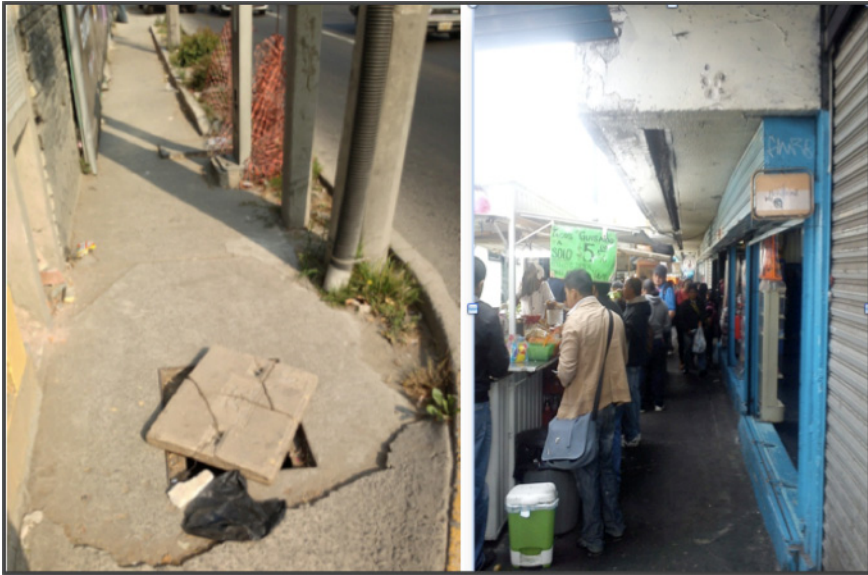
Fig. 2. Infrastructure and sidewalks problems
