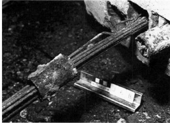
Fig. 11 Corrosion of longitudinal tendons at joint (Woodward and Williams 1988)
