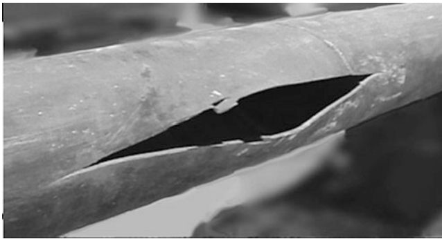
Fig. 10 Longitudinal failure in a boiler pipe
