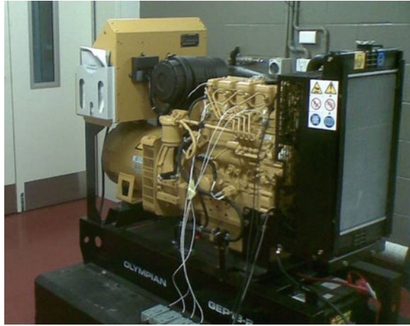
Fig. 38.4 The diesel fault test rig
