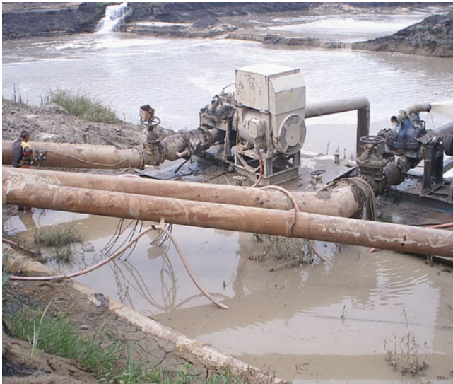
Fig. 1 Flooding water discharge pump
