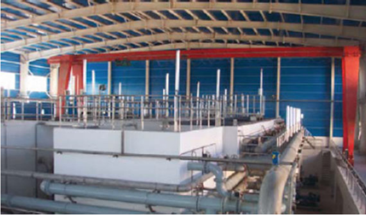
Fig. 11 Wastewater treatment in Beijing Olympic Park (GE Water Treatment Technologies) [9, 29]
