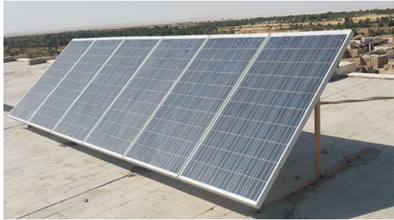
Fig. 46.2 Polycrystalline PV a top of school
