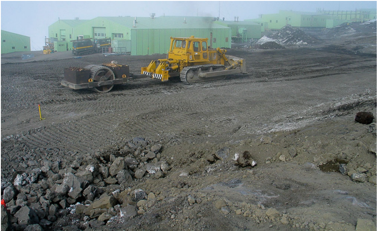
Fig. 15.3 Earth moving equipment preparing a building site adjacent to Scott Base is an example of the most intense scale of disturbance that occurs near permanent bases (Photo Taken January 2004 by Megan Balks)
