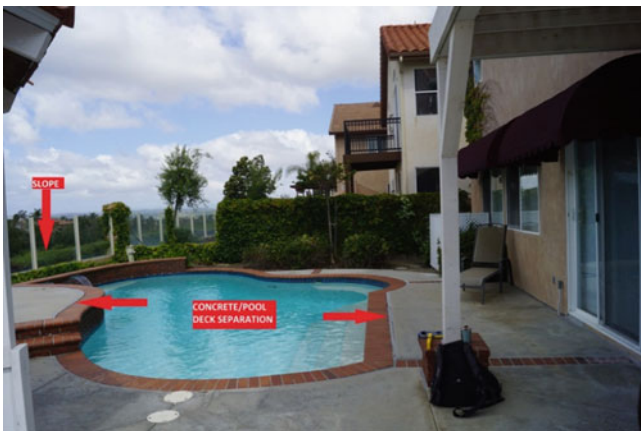
Fig. 6 Separation of pool walls from the floor slab—identified during the field visit
