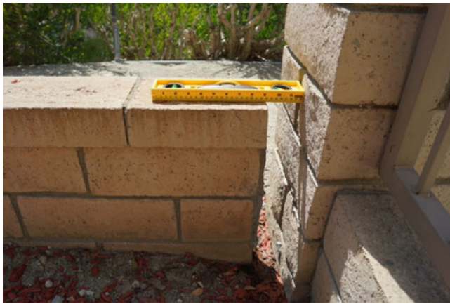
Fig. 5 Separation of compound wall from the main building—identified during the field visit
