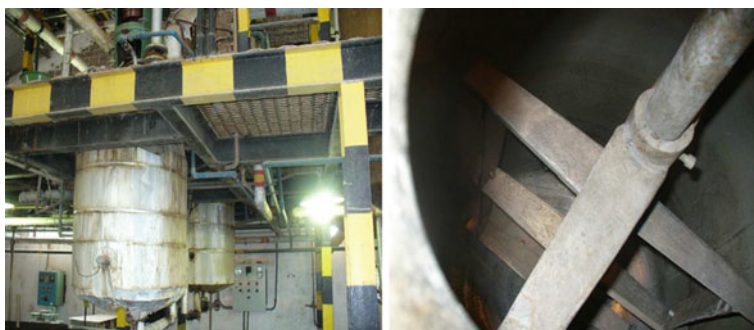
Fig. 11.7 Picture of the 350L reactor, where a diluted sulfuric acid pretreatment of sugarcane straw were performed for production of second-generation ethanol
