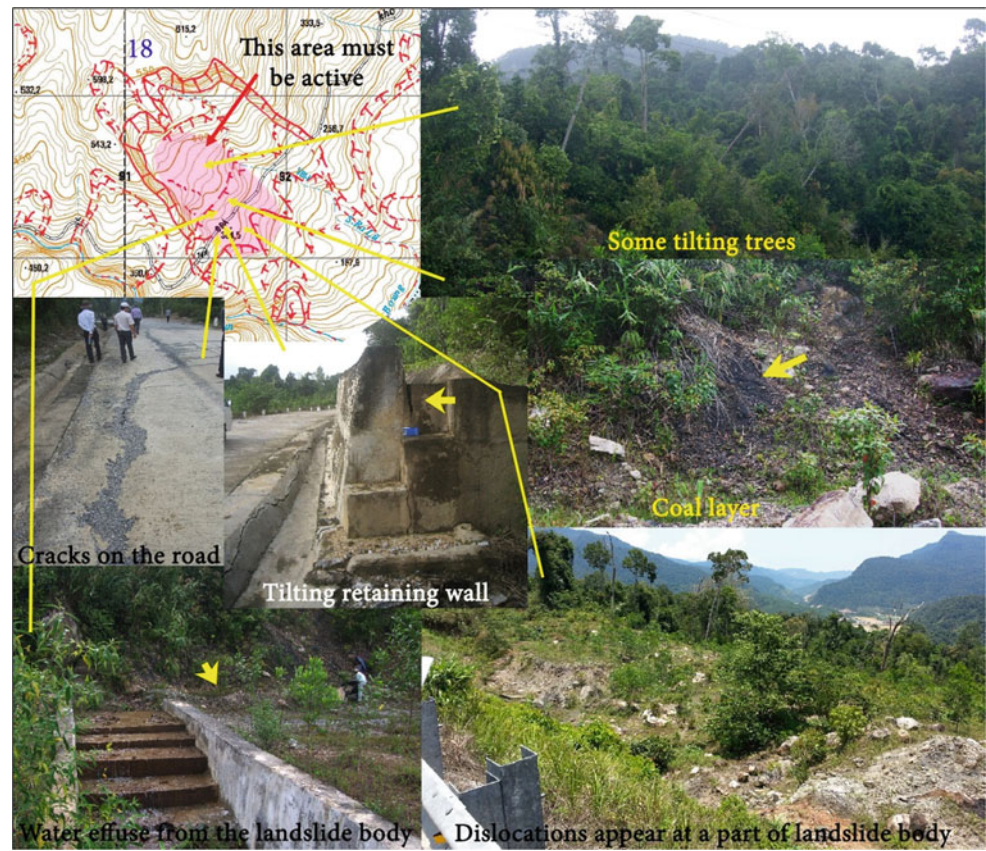
Fig. 6 Some evidence of landsliding was observed at a part of landslide No. 18
