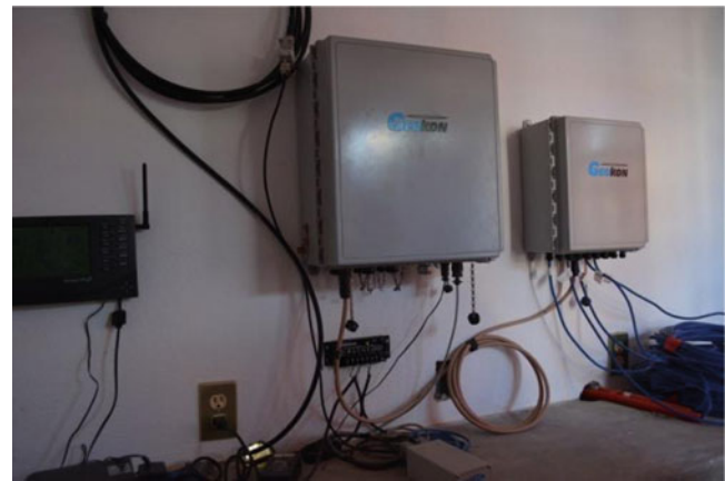
Fig. 10 Monitoring system inside of the booth
