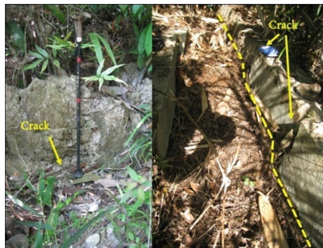
Fig. 5 Cracks on top of slope and concrete ditch at landslide No. 21
