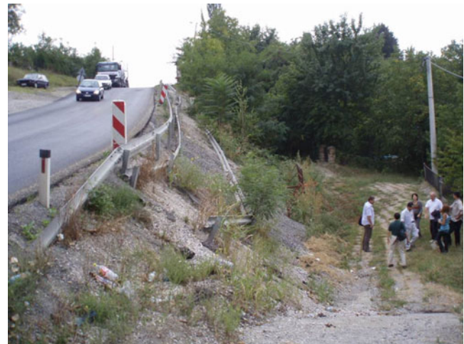
Fig. 5 Deformation on road M-19
