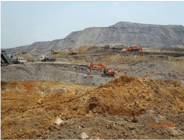
Fig. 5 Dump site area after the landslide
