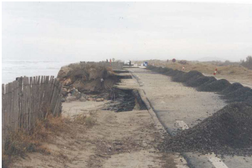
Fig. 4.19 Recurrent erosion impacts on the coastal road
