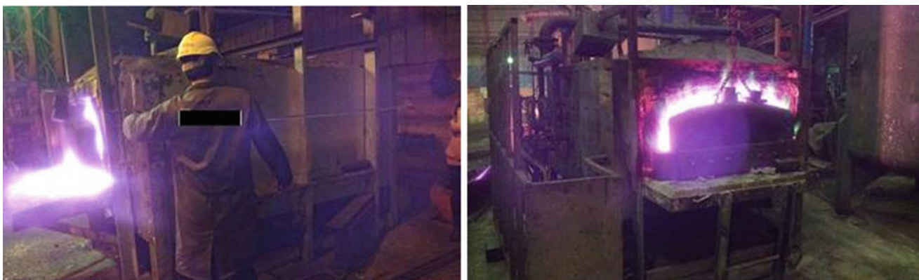
Fig. 96.2 An operating natural gas fired furnace
