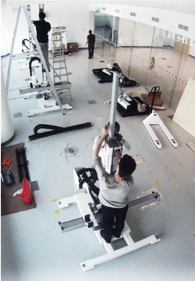
Fig. 4 A simple pulley is used for installation and height adjustments; the vertical axis is modularized into five segments (Gramazio and Kohler, FCL Singapore, 2012)
