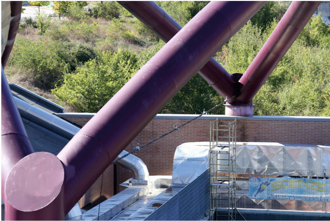
Fig. 30.4 Installation of the prototype of monitoring system on one of the cables of a sample arch steel roof
