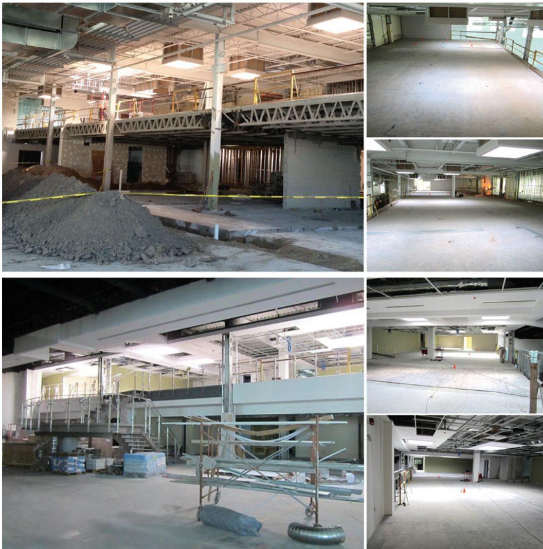
Fig. 6.1 Photos of the test floor during early renovation/demolition ( top ) and partial fit-out ( bottom )
