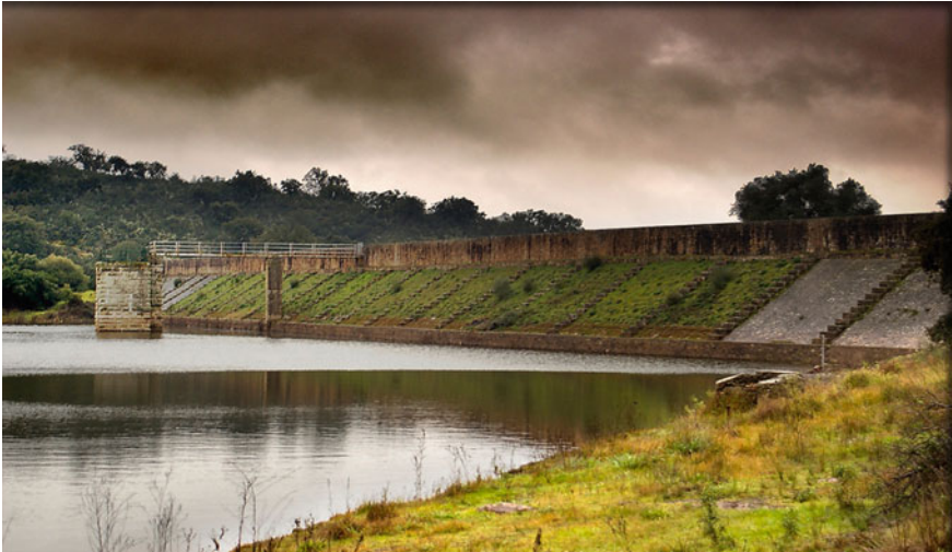
Fig. 1.3 The Cornalvo dam, Spain—1,500 years young—a well maintained dam can be operated for many years for sustainable water supply. The Cornalvo dam in Spain was built by the Romans almost 1,500 years ago and it is still fully functional (Wikipedia 2013)
