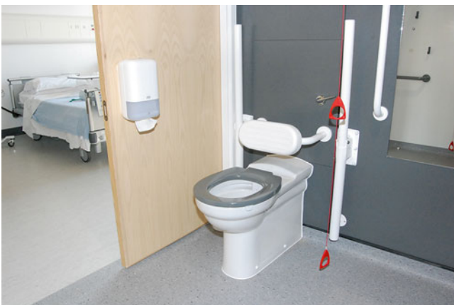
Fig. 13.6 Floor mounted toilet
