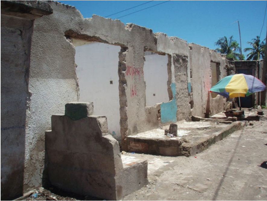
Fig. 10.4 Abandoned houses in local areas destroyed by floods (Picture: Dorthe Hedensted Lund 2013)
