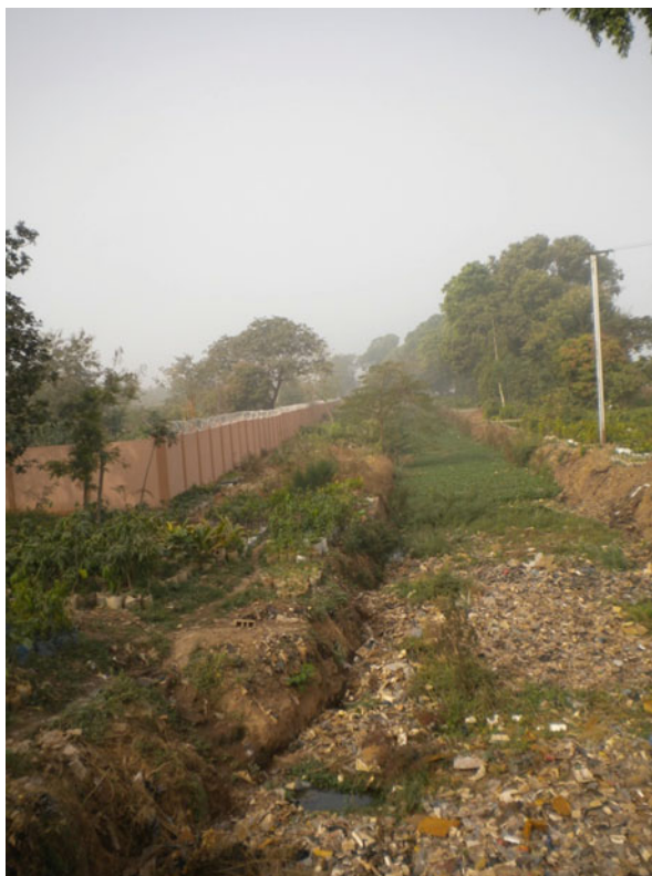
Fig. 12.4 Sewer clogged by waste in the city of Ouagadougou (Picture: Hamidou Touré 2011)
