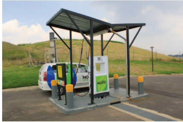
Fig. 15.4 Filling station of NOVO for upgrades landfill gas plant at the Sebenza landfill site. (Source: Hugo A., NOVO)
