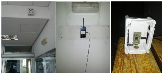
Fig. 3. Physical deployment in: entry of the building; second, boiler room; third, basement
