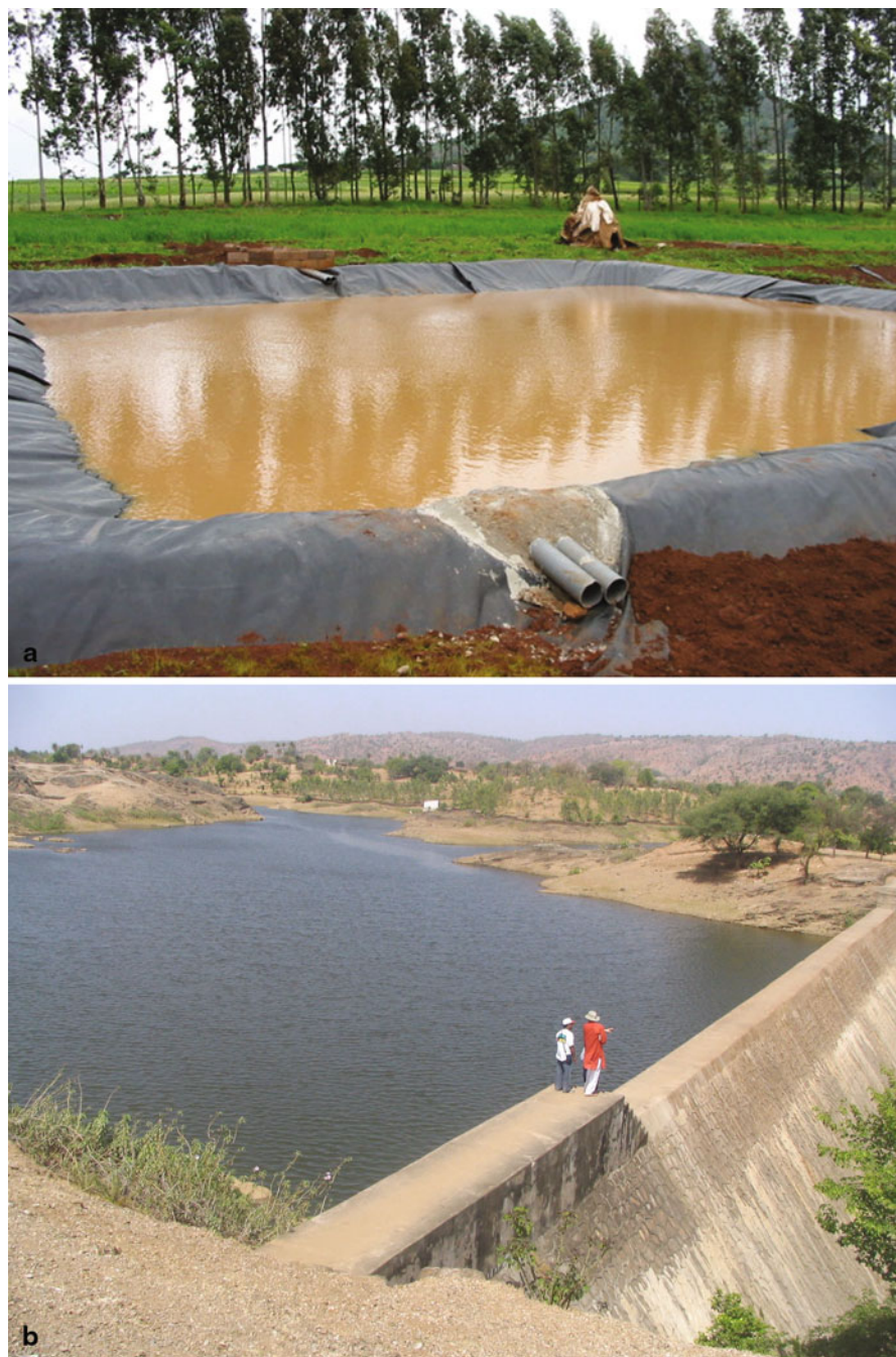
Fig. 28.2 a Water harvesting pond in the Nile basin with inflow and outflow structures. b Runoff collection pond in India with overflow weir
