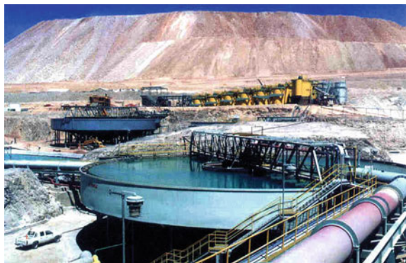
Fig. 1.8 View of a conventional thickener for copper tailings
