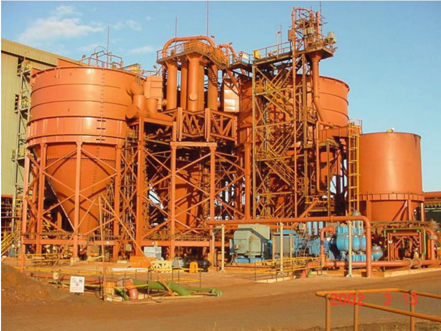
Fig. 8.17 View of paste thickeners. (courtesy of Eimco process equipment)
