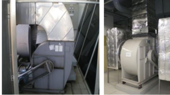
Fig. 2 Air supply blower
