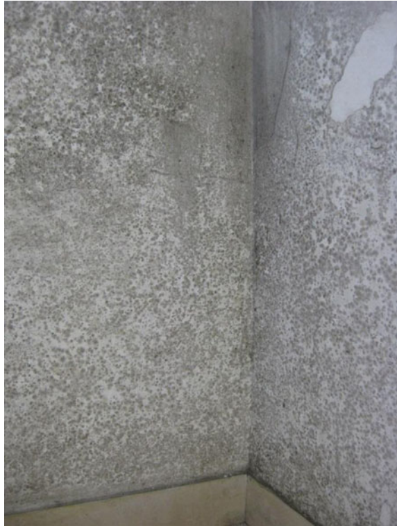
Fig. 4.2 Massive proliferation of mould inside a building
