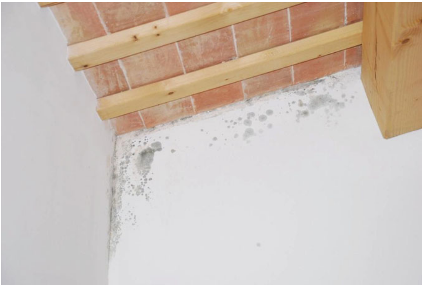
Fig. 6.2 Example of mould formation in a renovated building whose walls had been recently insulated: the concrete beam of the roof forms a thermal bridge that was not correctly treated
