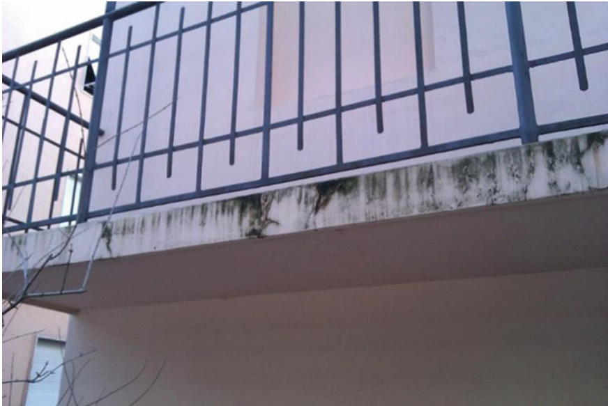
Fig. 3.4 A typical algal growth on a balcony caused by wind-driven rain. The water run-off carries dirt and spores from the balcony slab causing the formation of typical vertical stripes
