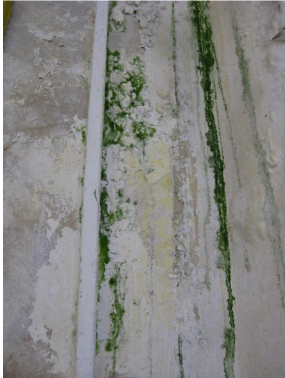
Fig. 3.7 Evident damages on a building surface due to microorganism colonisation
