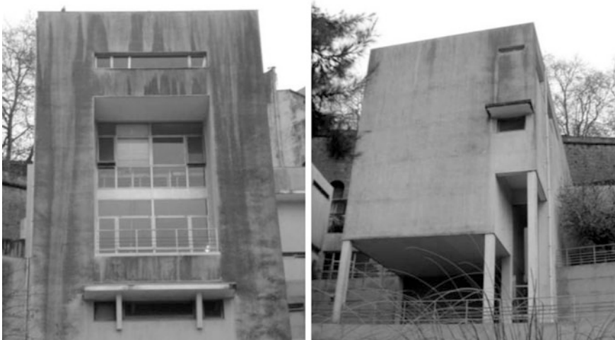
Fig. 6.3 ETICS defacement due to biological growth (buildings located in Porto, Portugal). Reprinted from Barreira and de Freitas (2013), copyright 2013, with permission from Elsevier
