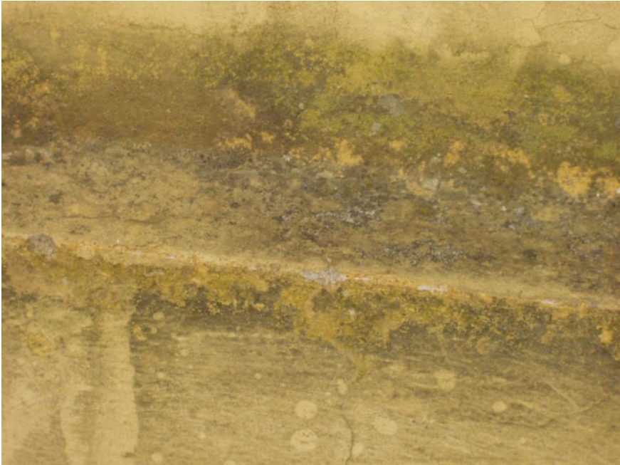
Fig. 3.1 Example of biofilm with traces of different colours ( black, green, yellow ) extend over the entire surface of a building façade
