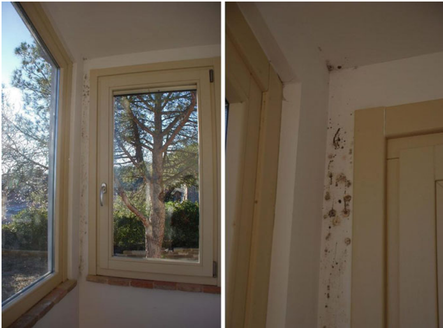
Fig. 6.1 Example of a typical mould formation after the replacement of single glazed windows by new tight windows. View of the new windows installed (on the left ) and detail (on the right )
