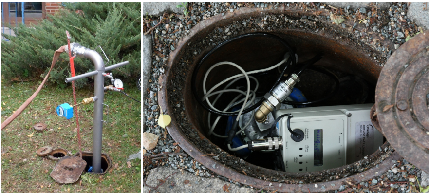
Fig. 1 On-situ continuous measurement of flow and Fig. 2 On-situ measurement of hydrodynamic pressure – underground hydrant hydrodynamic pressure
