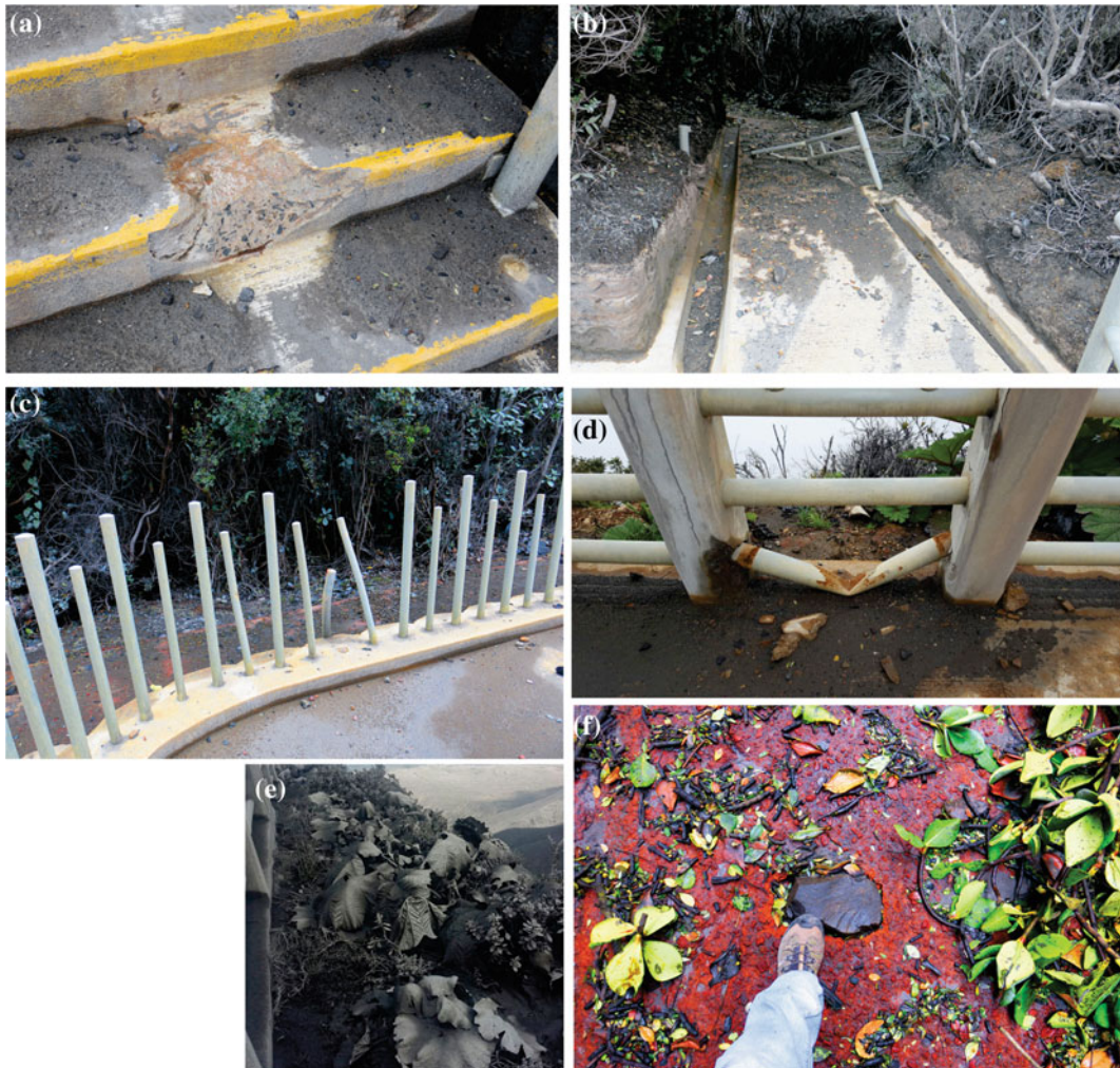
Fig. 24 a The recently restructured sector of the tourist mirador was damaged most by the April 2017 eruptions. The ramps and stairs were destroyed by the impact of bombs. b , c and d Examples of the damage to metallic structures in the mirador area. e Vegetation (“poor man’s umbrellas”) at the tourist mirador were “burned” by
