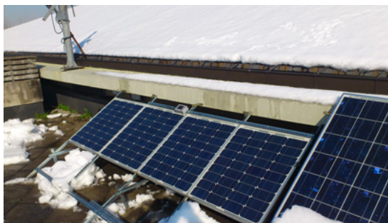
Fig. 3. ATERSA A55 photovoltaic modules
