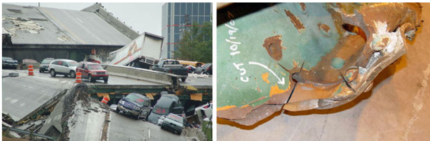
Fig. 13.31 Photo on left of the Minneapolis bridge collapse; photo on right showing fracture in gusset plate
