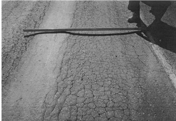
Fig. 13.7 Photograph of asphalt pavement that is both rutted and cracked
