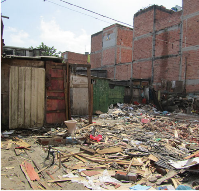
Photo 4.16 Favela Leste – section four – the beginning of the demolition of the favelinha 2013
