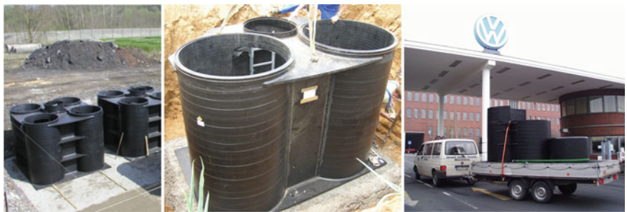
Fig. 4 Alternative designs of containerised PE-HD lysimeter stations (from left to right —4-fold, 2-fold and 1-fold lysimeter station during installation)
