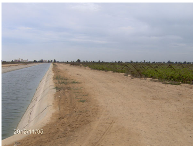
Fig. 9 The main irrigation canal is lined using the agricultural water management near the grapevine in Nubaria district, Egypt (Photo by H. El-Ramady)
