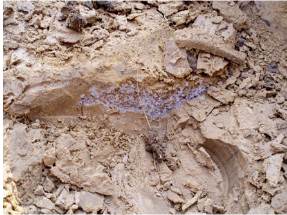
Fig. 4 Segregation-ice caused by the migration of water in the pit
