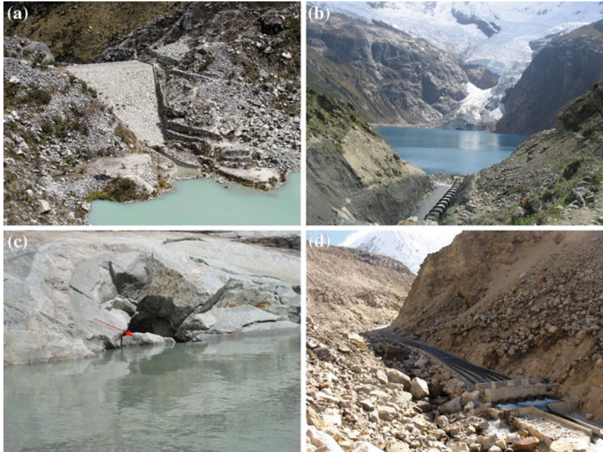
Fig. 9 Examples of remedial works. Part a shows artificial dam and concrete outlet of lake Laca in the central part of the Cordillera Blanca; dam freeboard is 12 m. Part b captures ongoing work on the dam of lake Rajucolta in 2004. Part c shows the entrance to the tunnel excavated in the bedrock dam of lake No. 513 ( red arrow ). Part d shows six siphons installed in fall 2011 to drain and lower the water level of lake Palcacocha
