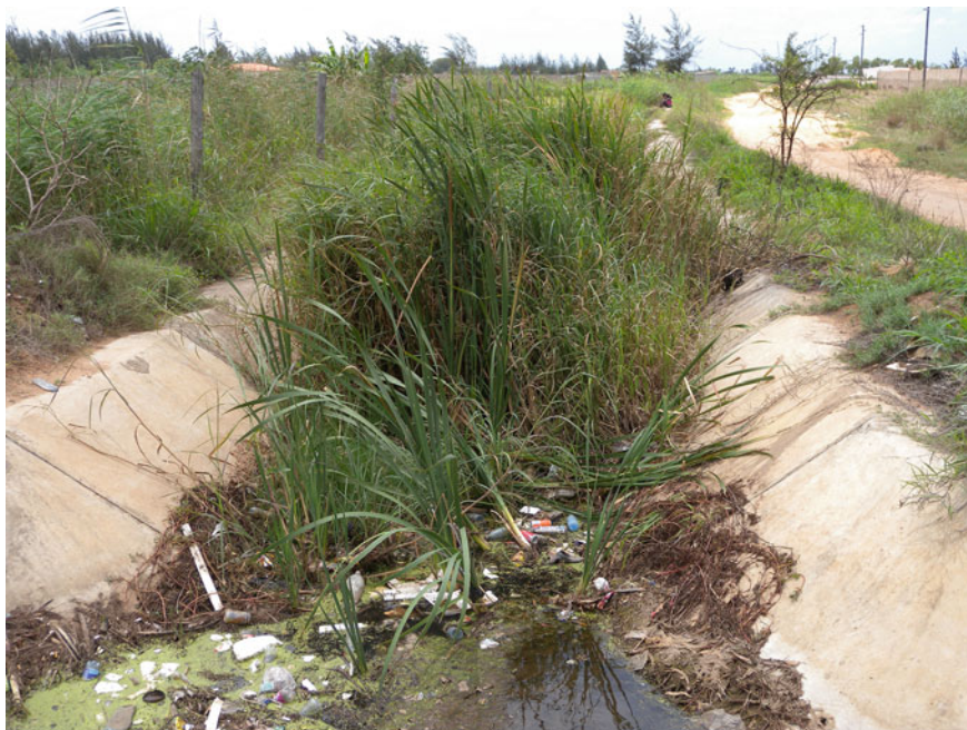
Fig. 13.5 Maputo, KaMavota district, 3 Nov. 2011. Stormwater drainage along Dona Alicia Street with efficiency compromised by vegetation (Tiepolo 2011)
