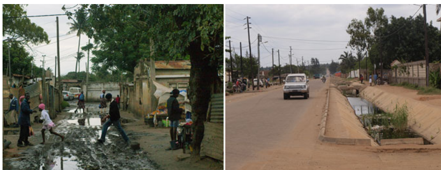
Fig. 12.4 Left Maputo, Mafalala bairro, Nov. 2011. People walking along an unpaved flooded road; Right Maputo, Costa do Sol bairro, Rua Engenheiro Santos Resenoe, Nov. 2011. Paved road with a drainage canal (E. Ponte)
