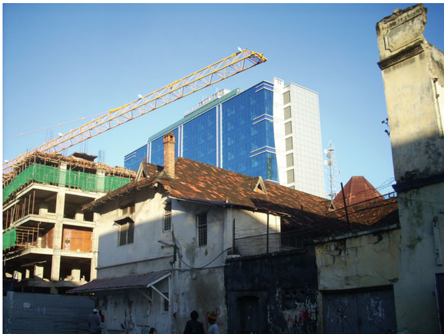
Fig. 1.3 Densification under way in a central area of Dar es Salaam (photo by Silvia Macchi)
