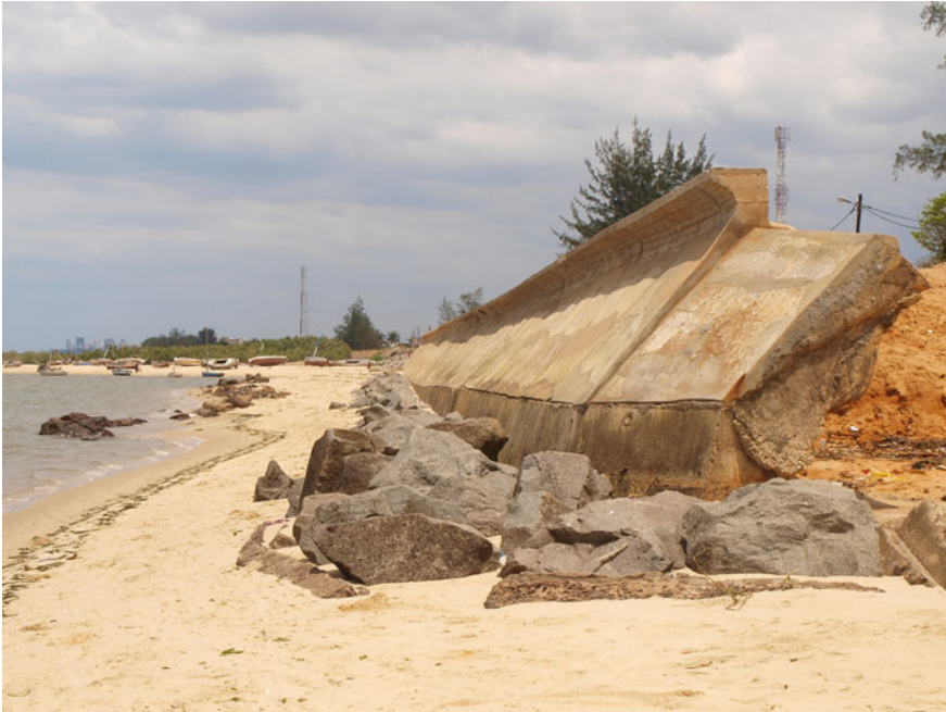
Fig. 13.4 Maputo, district 4, 3 Nov. 2011. Sea wall in the Costa do Sol neighborhood (Ponte 2011)
